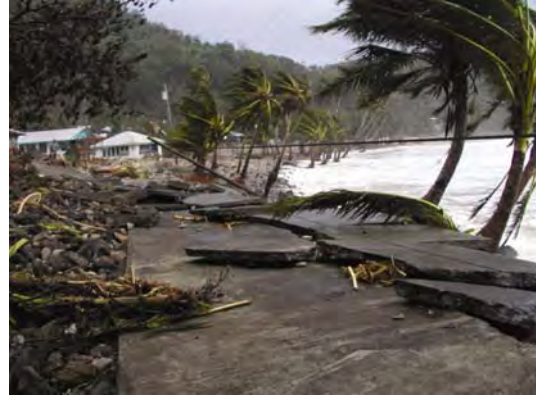
Damage to Onenoa in 2004 (Cyclone Heta).
