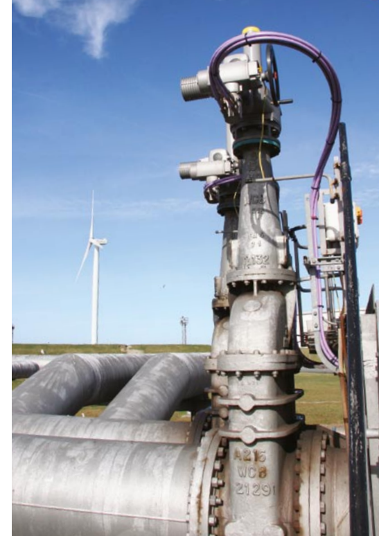
BP Refinery in Rotterdam servo-drive on PROFIBUS
